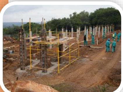
Top to bottom: The new weeds quarantine and nursery buildings under construction
