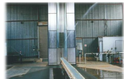
Sprinkler test bench
