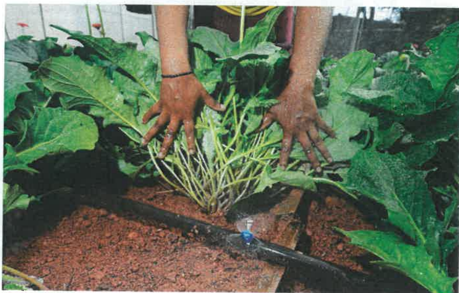
Installation, spacing and operating pressure are some of the important aspects that require attention when installing an irrigation system.
